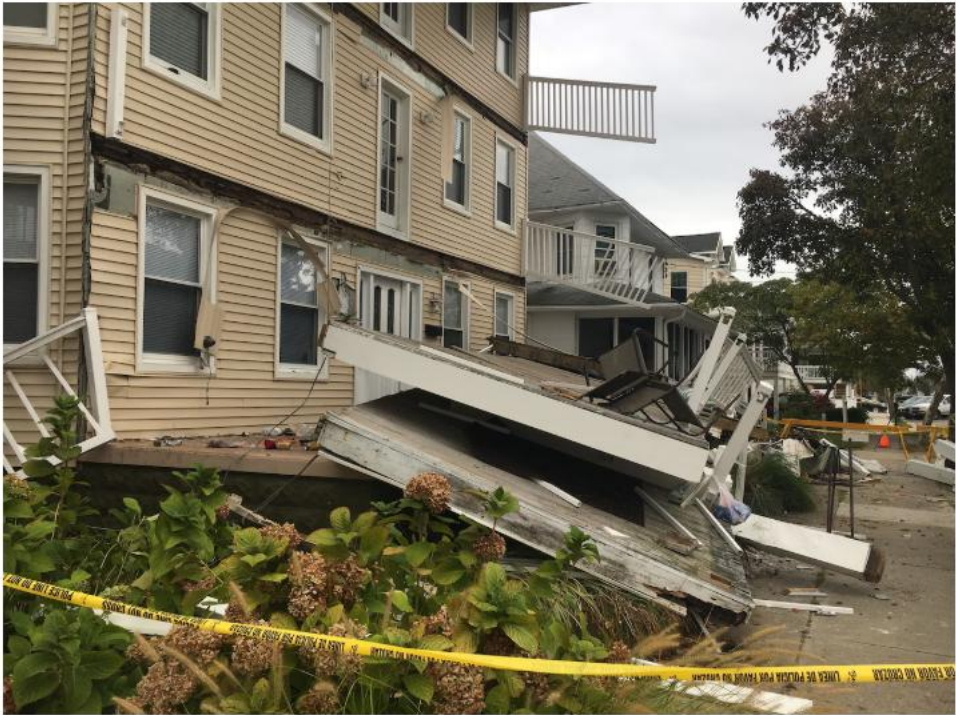
Multiple decks collapsed Saturday, Sept. 14, 2019, in Wildwood during the annual firefighters weekend. This is a photo of the aftermath, taken on Sunday, Sept. 15. Tim Hawk | NJ Advance Media for NJ.com
